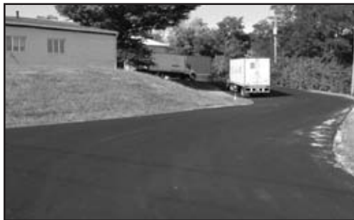
Replacing the driveway to make it safer for trucks and other vehicles was one of the major projects Shared Harvest Foodbank had to undertake in 2010.
